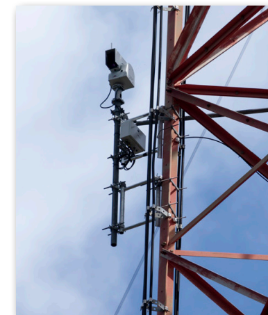
The Firewatch camera system is mounted to a City of Austin communications tower on Mount Larsen, just north of West Lake Hills. Camera images are relayed to our dispatch center using wireless radio signals.
