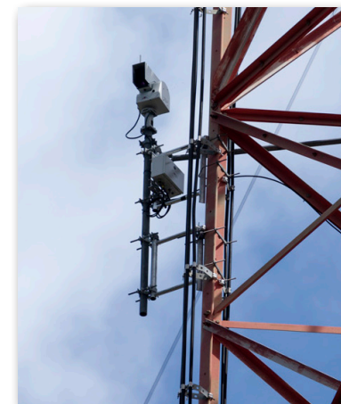
The Firewatch camera system is mounted to a City of Austin communications tower on Mount Larsen, just north of West Lake Hills. Camera images are relayed to our dispatch center using wireless radio signals.
